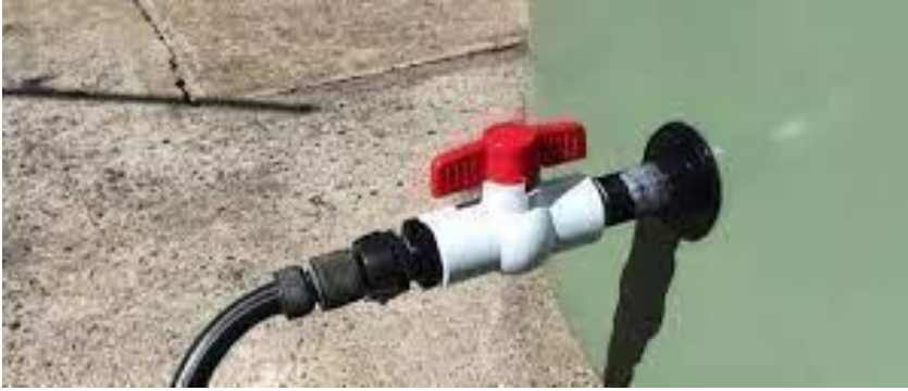
Watertight seal with attached ball valve on the side wall of a tank
