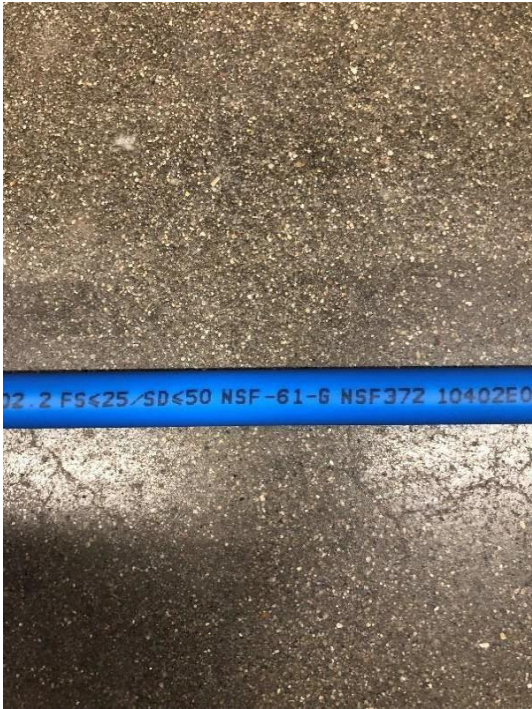
Blue potable PEX line with NSF label
