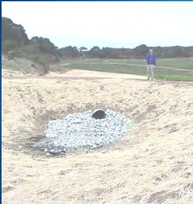
Rock Energy Dissipaters
