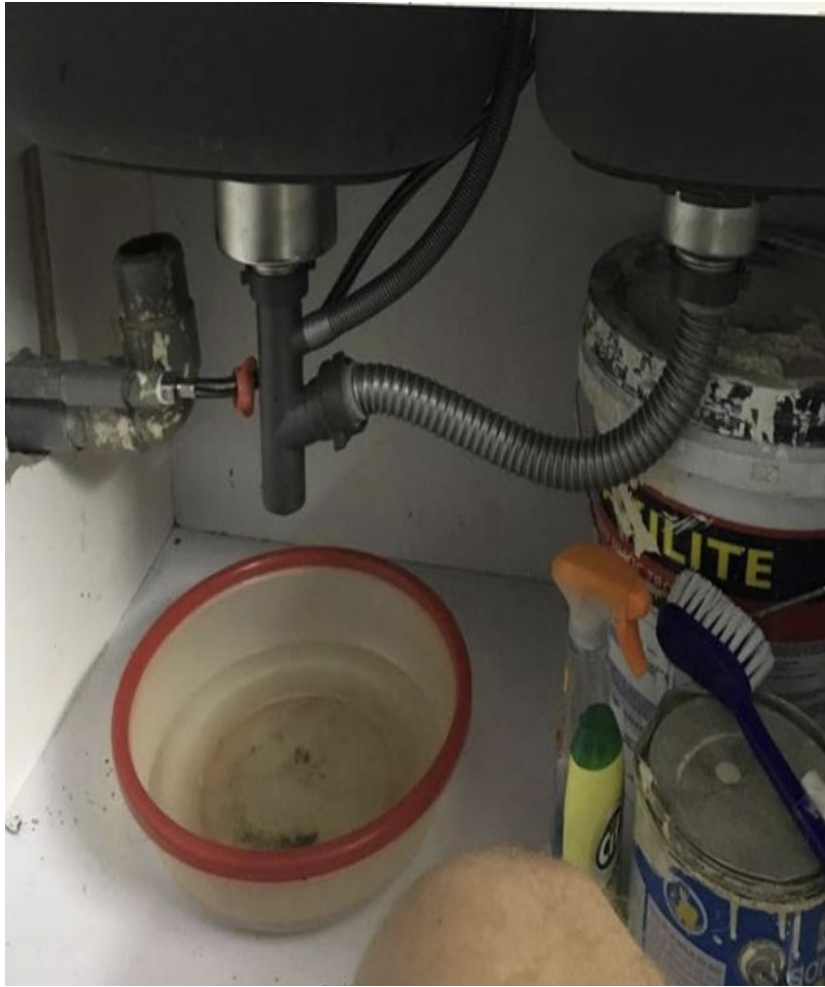
Bad: Open container, not appropriately containerized, spill potential is high, potential
