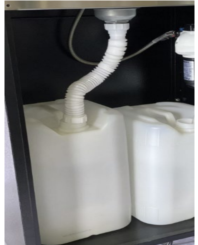
Good: Sealed container, minimal spill potential, easy removal and replacement.
