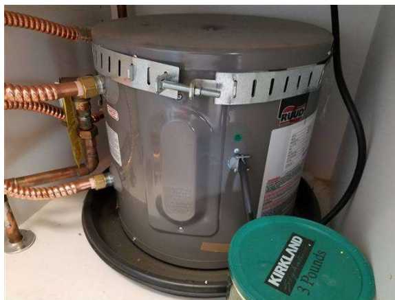
Six Gallon Electric Water Heater
