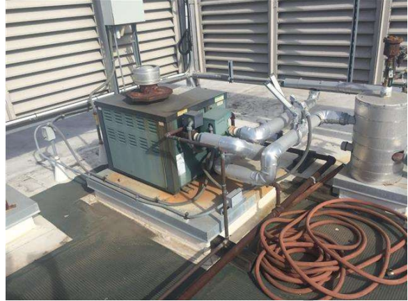
Natural Gas Fired Boiler
