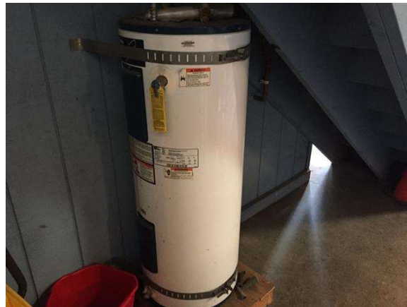
40 Gallon Electric Water Heater
