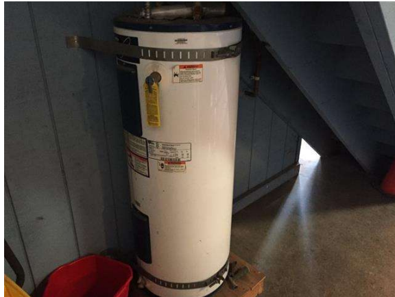
40 Gallon Electric Water Heater
