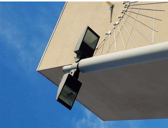
70 W Pole-Mounted MH Fixtures
