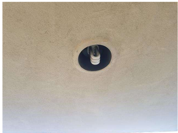
26 W CFL in Recessed Can Fixture
