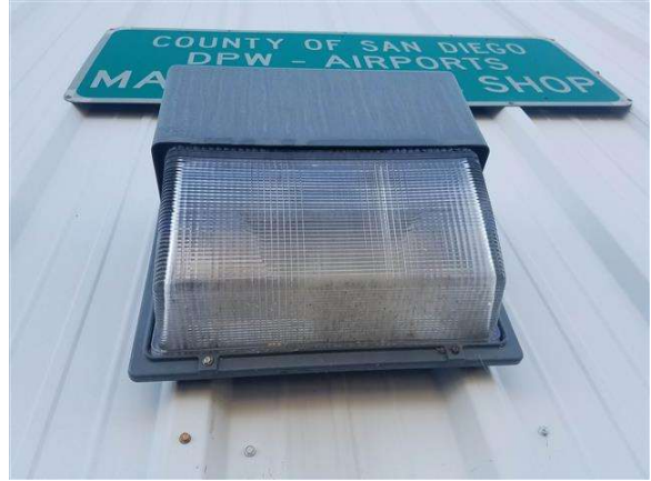
100 W Wall-mounted MH Fixture
