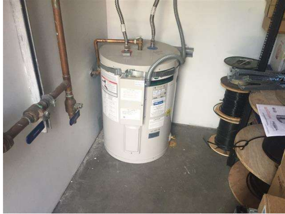
30 Gallon Electric Water Heater
