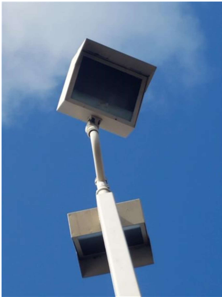
250 W HPS Pole-Mounted Fixture
