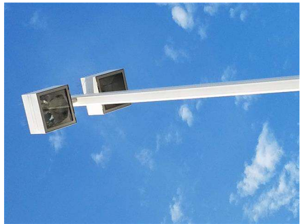
100 W Pole-Mounted HPS Fixtures
