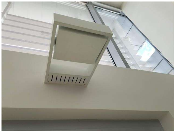
26 W CFL in Uplight Fixture
