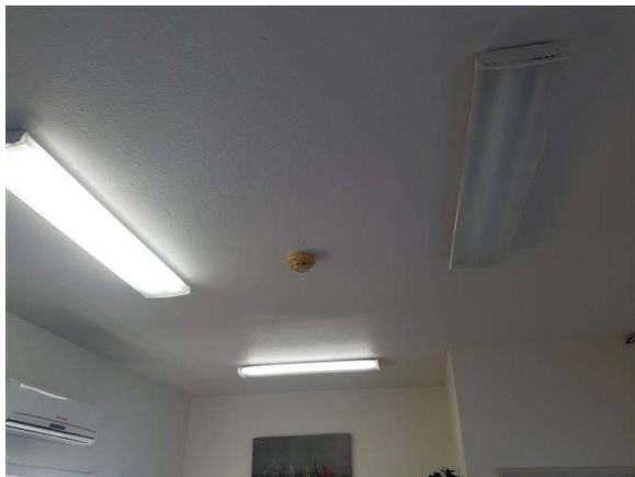
40 W 2-Lamp T12 Linear Fixtures
