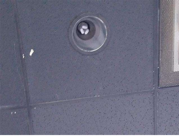
26 W CFL in Recessed Can Fixture
