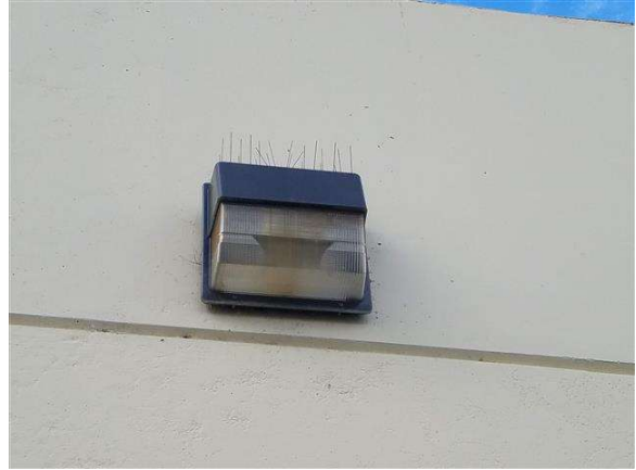
Wall-Mounted 100 W HPS Fixture
