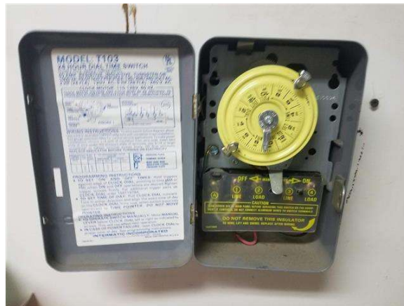
Electromechanical Timer for Exterior Lights
