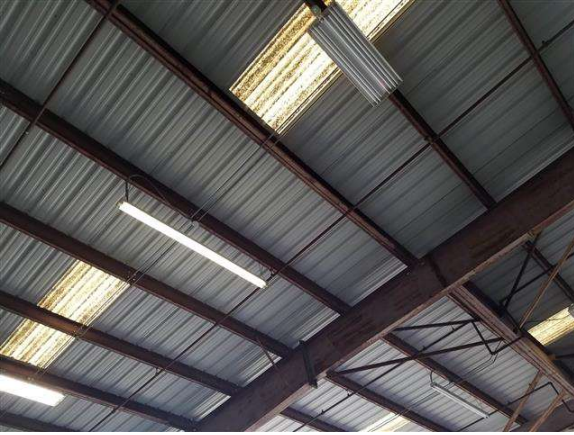
T12 and T8 Pendant Fixtures
