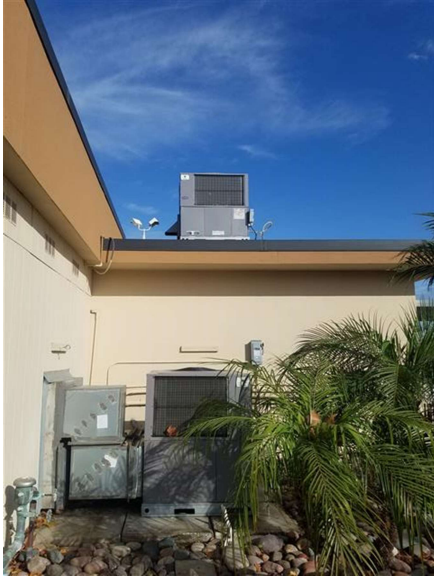
Packaged Rooftop AC Unit
