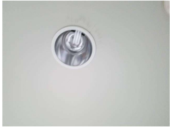
26 W CFL in Recessed Can Fixture
