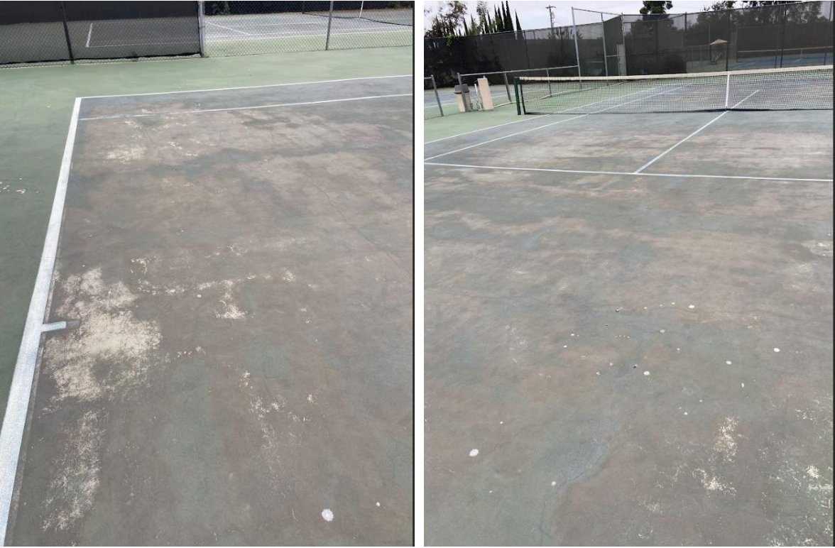
Figure 20 Several Courts in Need of Resurfacing – slip hazards.
