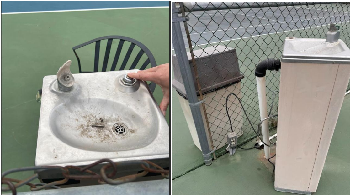
Figure 12 Broken & Dirty Water Fountains
