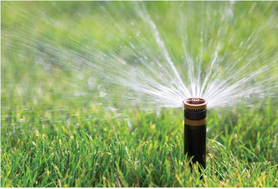
A sprinkler head only spraying on a landscaped area
