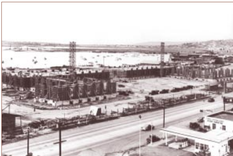
From the ground up: These photos are part of a series chronicling the progression of the building.
