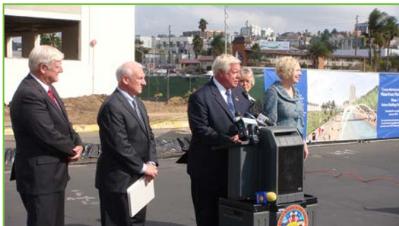
From left to right: Supervisor Greg Cox, Supervisor Ron Roberts, then-Chairman Bill Horn, Supervisor Dianne Jacob, and Supervisor Pam Slater-Price kick off the demolition of the J.B. Askew Building.
