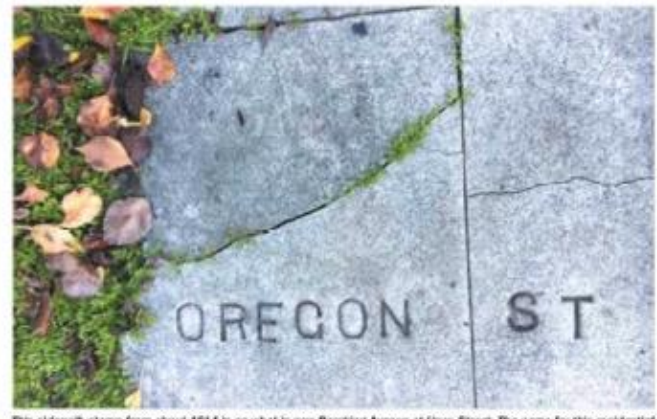
This sidewalk stems from about 1914 in what is now Pershing Avenue at Guas Street. The name for this residential
