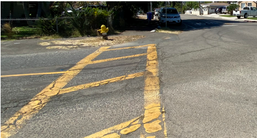
The high visibility crosswalks in Townsite are fading and should be restriped.
