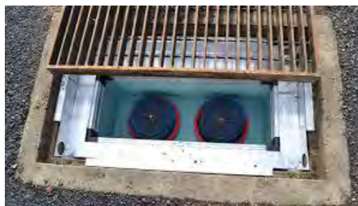
Photo 15: Catch basin with filtration system. This is an example of a modified storm drain inlet that includes a basin for capturing debris and a treatment system for reducing pollution before the water enters the storm drain. County of San Diego standards should be consulted for the exact design requirements for inlet and filtration system design when design drawings are prepared.
