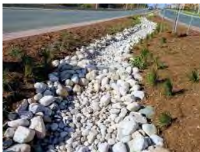
Photo 14: Alternative to landscape bioswale. In this case, mulch and rock can be used in the median, in curb extensions, and near the transit stops as an infiltration system to capture water that flows either from the new sidewalk areas or from the roadway.
