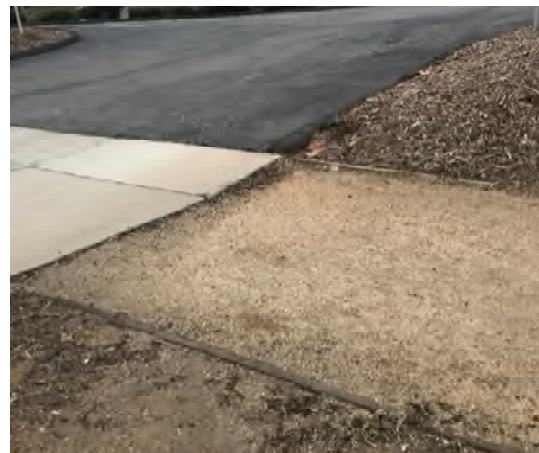
Figure 17: Example of trail erosion near concrete driveways.
