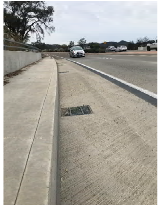
Figure 20: Class II bike lane with drainage inlet.
