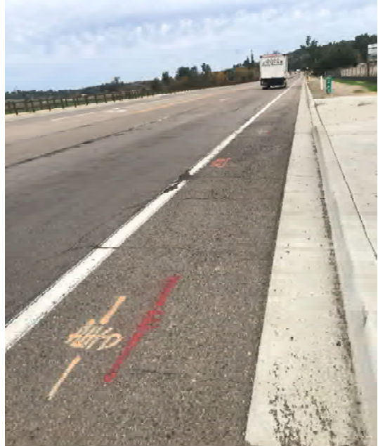
Figure 19: Class II bike lane with degraded surface.
