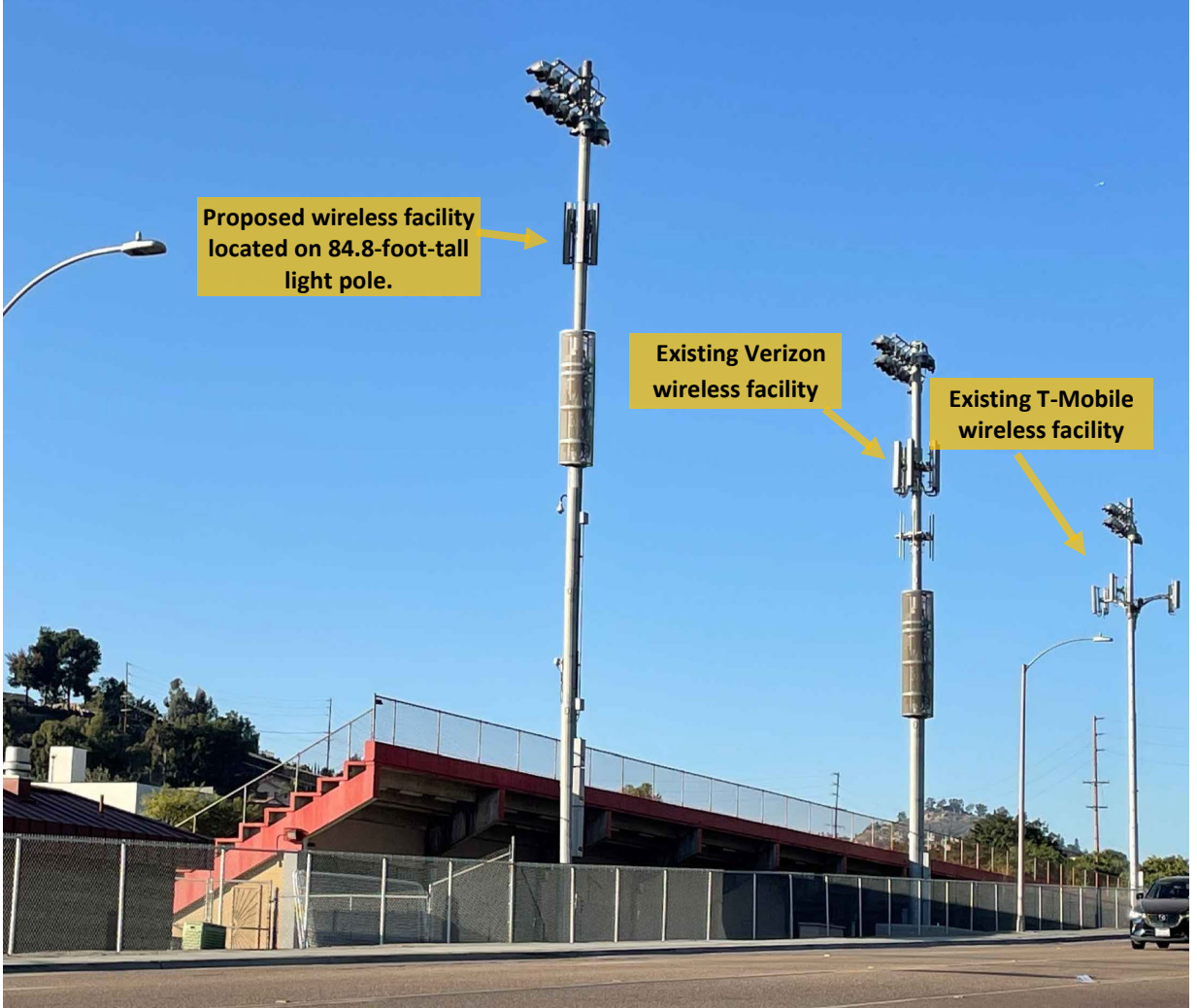
Figure 1: (Left) Proposed 84.8-foot-tall wireless facility, (Center) Existing Verizon 84.8-foot-tall wireless facility, and (Right) Existing T-Mobile 84.8-foot-tall wireless facility.
