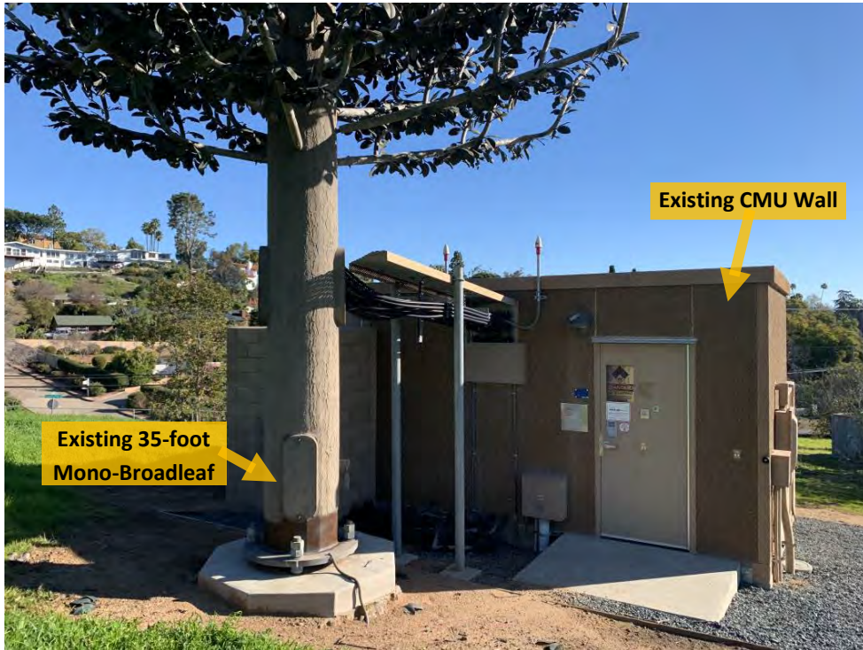
Figure 1: View of the existing mono-broadleaf tree and CMU wall, at base of project site.
