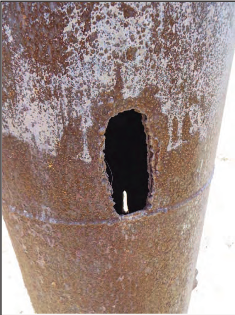
a. Torch Cut Hole in North Side of Pipe, Looking South (PR-05430-022)
