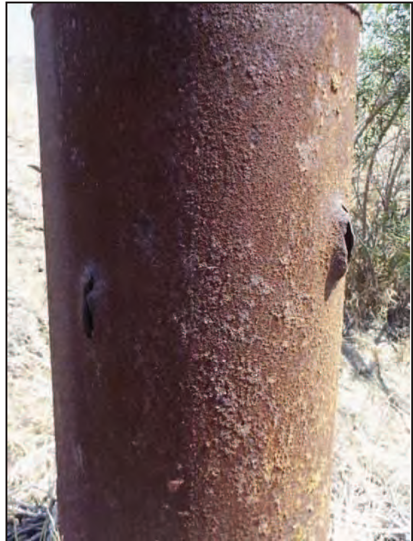
b. Close-up of Gashes in Pipe, Looking Northeast (PR-05430-023)
