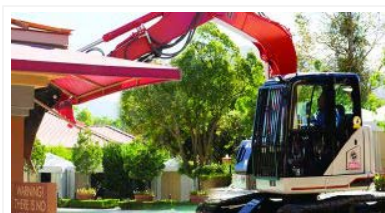
Pala Tribal Chairman Robert Smith drives an excavator through a brick kiosk building to make way for the new expansion.
