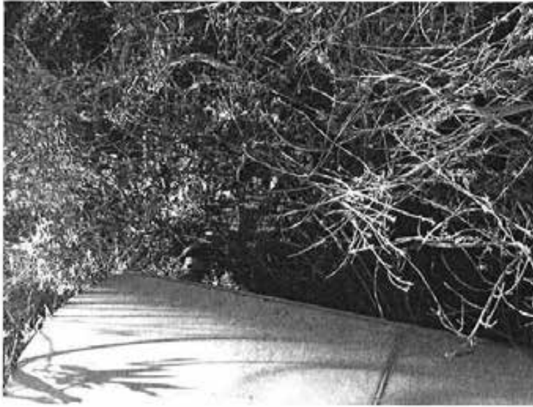
Tank, as found with two open ports, stained soil shows release.
