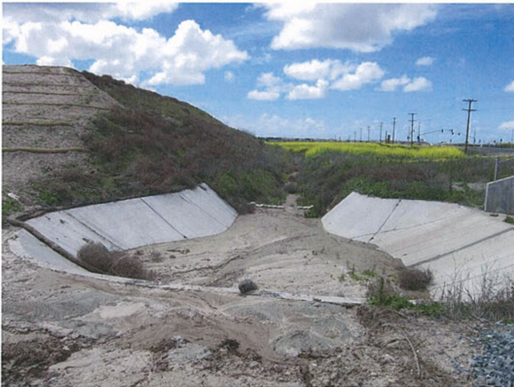
Figure 4. Looking Downstream (West) at Stilling Basin and into Upper End of Reach 1 (Point of Compliance Begins Here)
