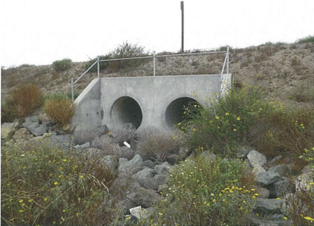
Figure 1. Double 60-inch RCP Outlets at POC 1
