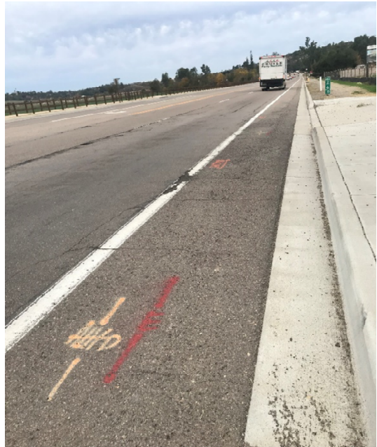
Figure 19: Class II bike lane with degraded surface.
