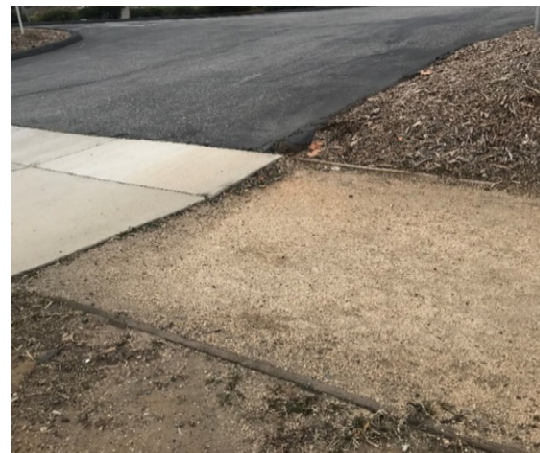
Figure 17: Example of trail erosion near concrete driveways.
