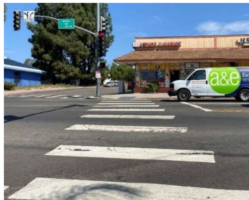
Figure 2: Existing crosswalk at Mission Road and Main Avenue show deteriorating pavement markings
