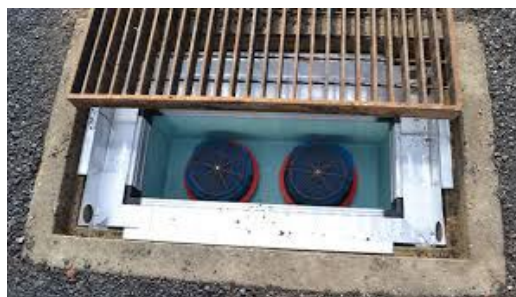
Photo 15: Catch basin with filtration system. This is an example of a modified storm drain inlet that includes a basin for capturing debris and a treatment system for reducing pollution before the water enters the storm drain. County of San Diego standards should be consulted for the exact design requirements for inlet and filtration system design when design drawings are prepared.
