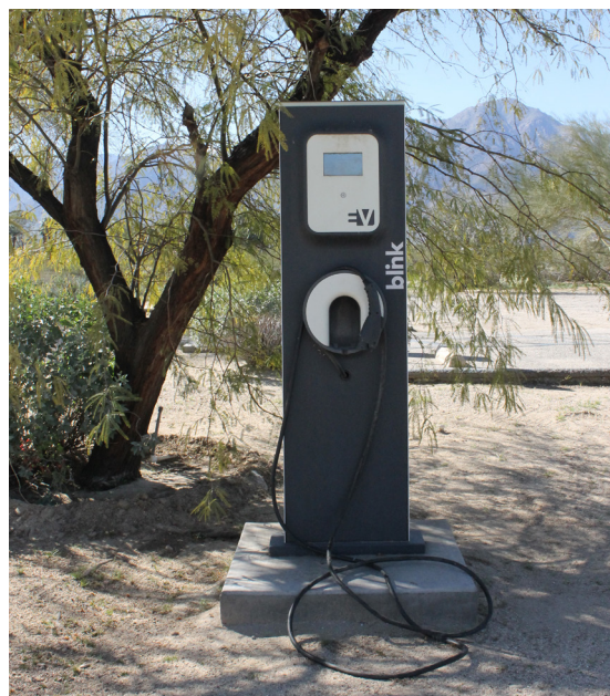
Local EV charging station in Borrego Springs.
