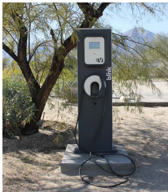
Local EV charging station in Borrego Springs.
