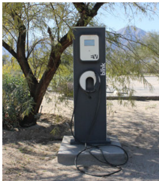
Local EV charging station in Borrego Springs.
