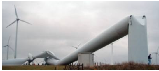
Figure E.9.2: Structural failure in western Germany.
