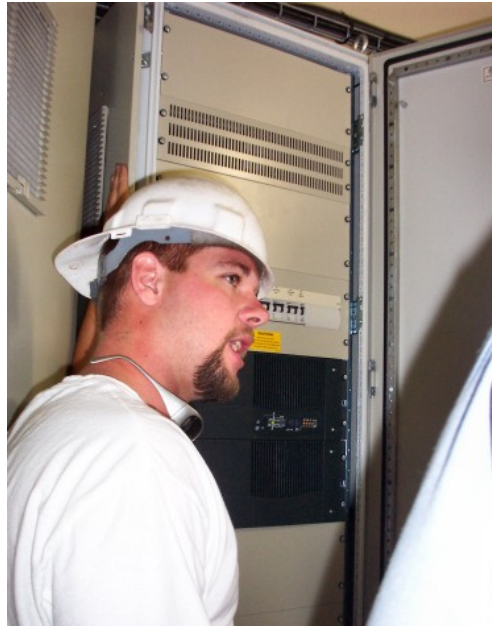
Figure C.1: Chris, a Vestas employee, explains how remote monitoring works while inside the turbine.
