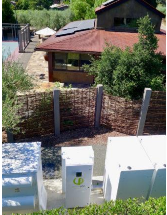
This LFP battery with inverter charge controllers, power electronics and system management was installed in a NEMA 3R outdoor-rated box, away from livable spaces, just in the off-chance of an accident.
