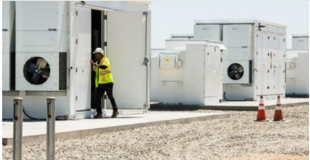
This large-scale lithium battery installation in California shows the ventilation systems used to keep batteries at a consistent temperature to prevent thermal runaway. (Photo by Dennis Schroeder / NREL)
