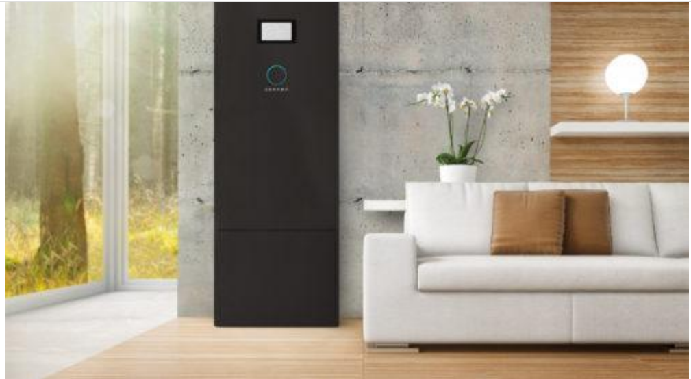
There may be adequate airflow to this energy storage system, but a safer alternate installation site is outside or in an unoccupied utility space.
