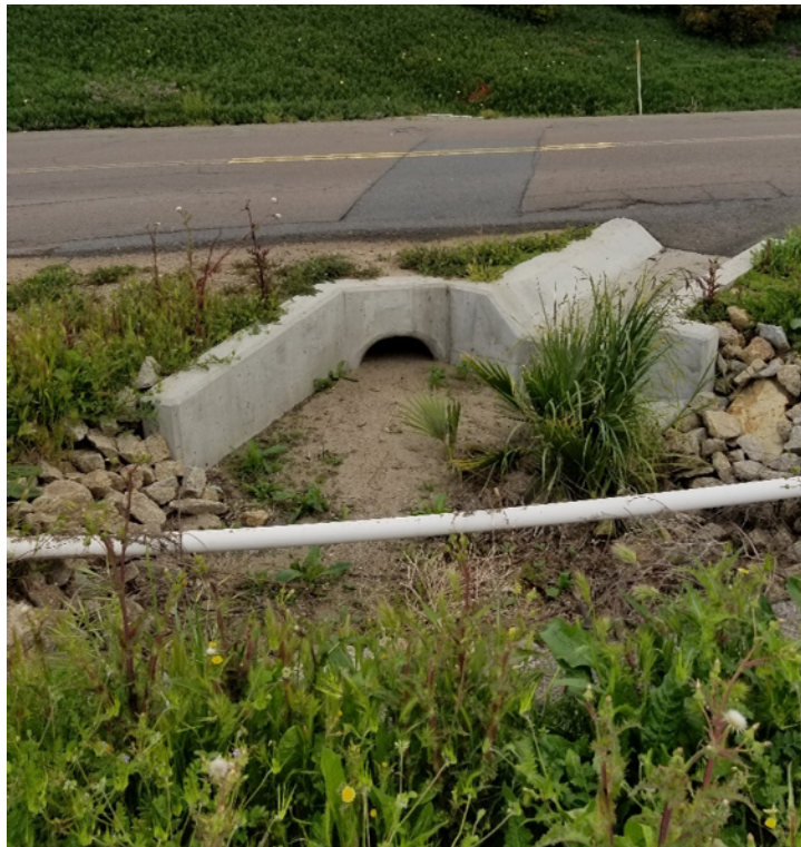
Photograph 14: View of concrete storm water drainage structure along Buena Vista Drive, looking east.
