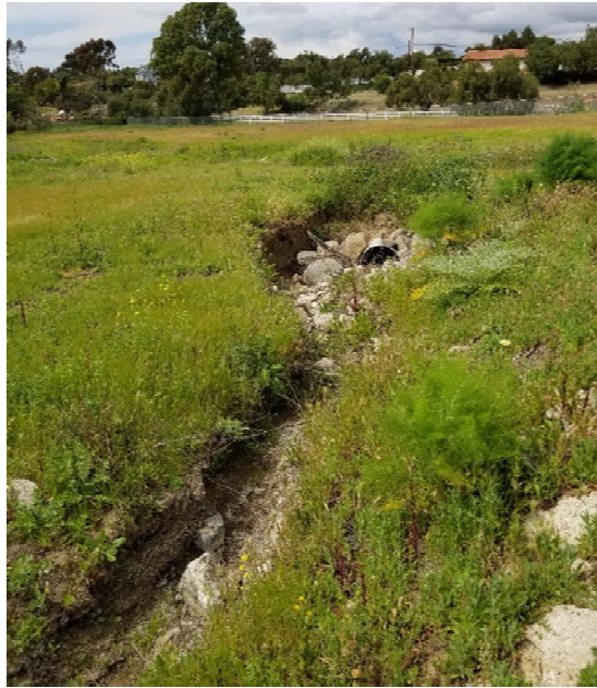
Photograph 17: View of north-south trending unlined drainage channel on the western portion of the site, looking north.
