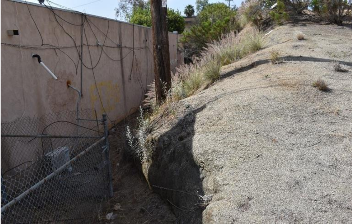
Photograph 6 Steep Drop-Off On The Eastern Side of the Project Area, View Southeast
