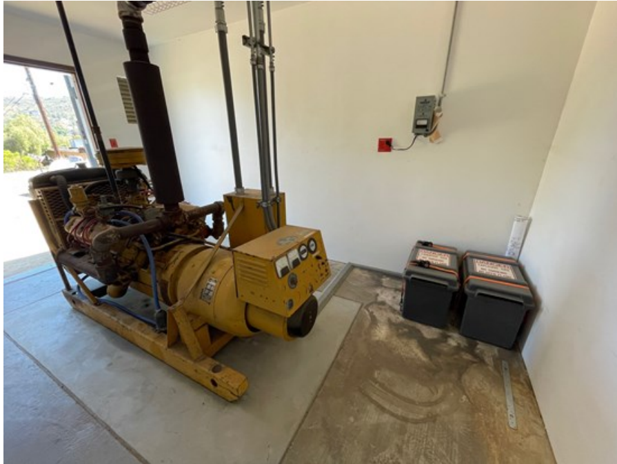
15. Emergency generator and lead-acid batteries.
