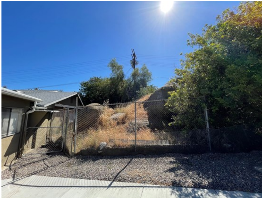
34. Transformers on adjoining property to the east.
