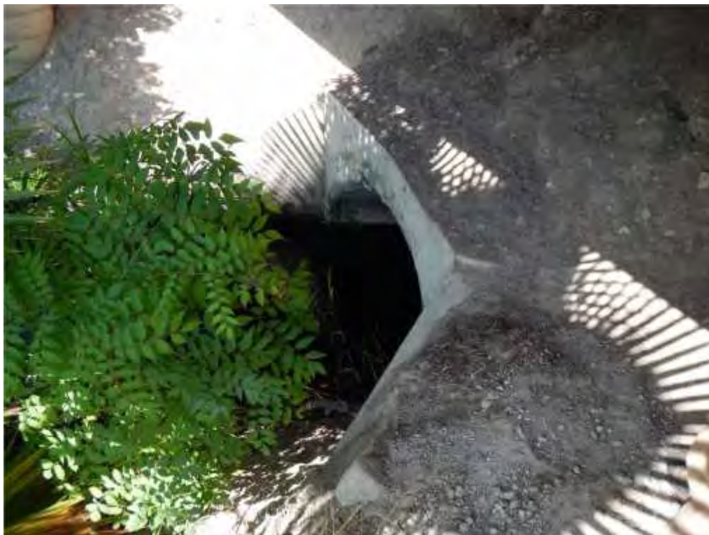
Photograph 1 – View of culvert inlet immediately upstream of the project boundary in the northern extent of the project site.
