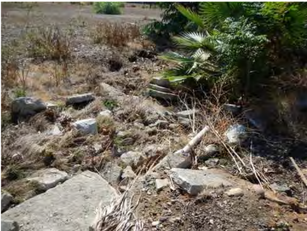
Photograph 10 – View of Drainage 1 looking downstream/southeast. Note debris and concrete in channel.
