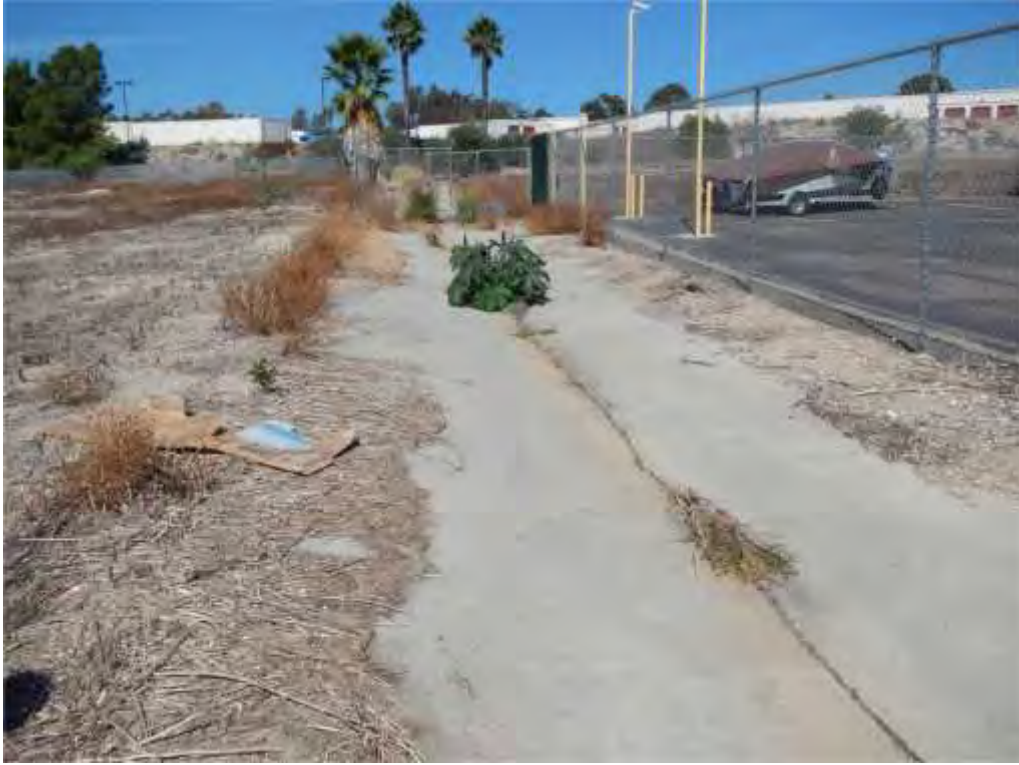
Photograph 17 – View of non-jurisdictional concrete v-ditch along eastern border of project site, looking upstream/north.
