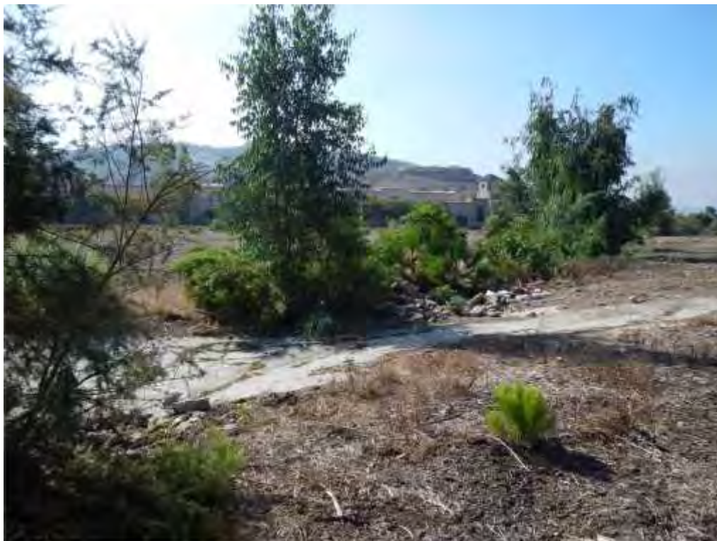
Photograph 7 – View of cement crossing that intersects Drainage 1, looking downstream/south. Eucalyptus trees, Mexican fan palms, castor bean, and other non-native vegetation dominate the feature.
