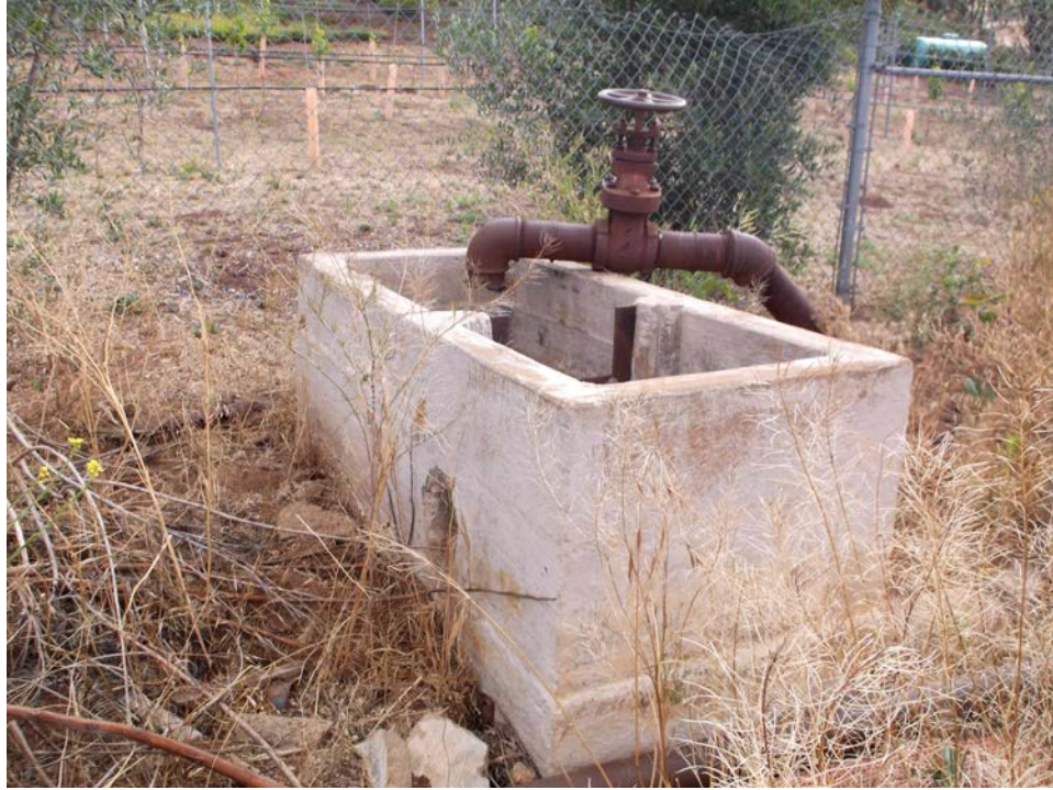
Figure 6. Valve for orchard irrigation system, facing east.
