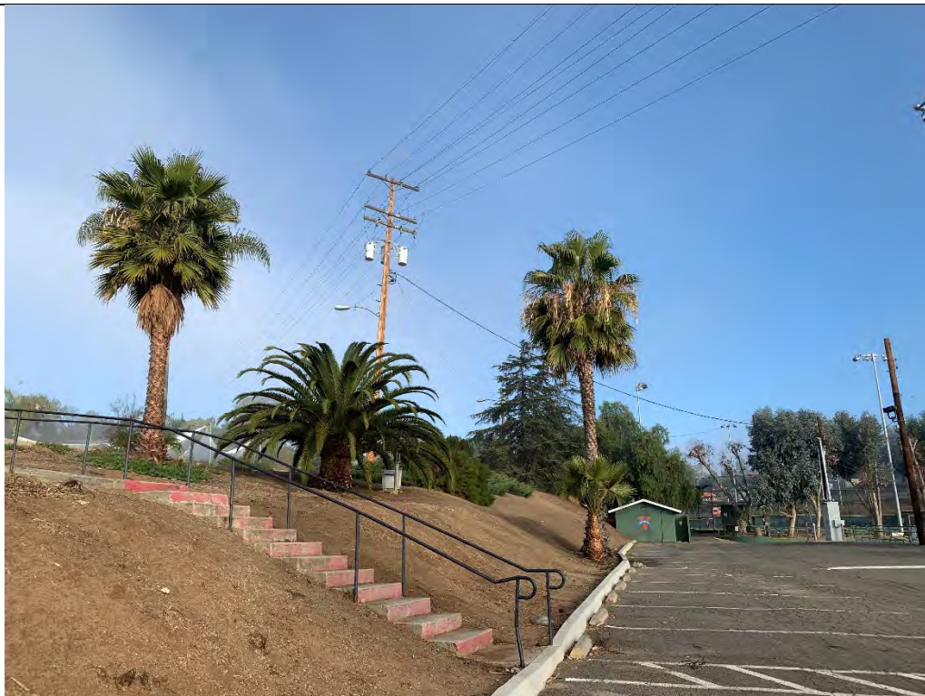
Photo #6 View of pole mounted transformer and overhead electrical lines located in the southern portion between the Subject Property and adjacent church.
