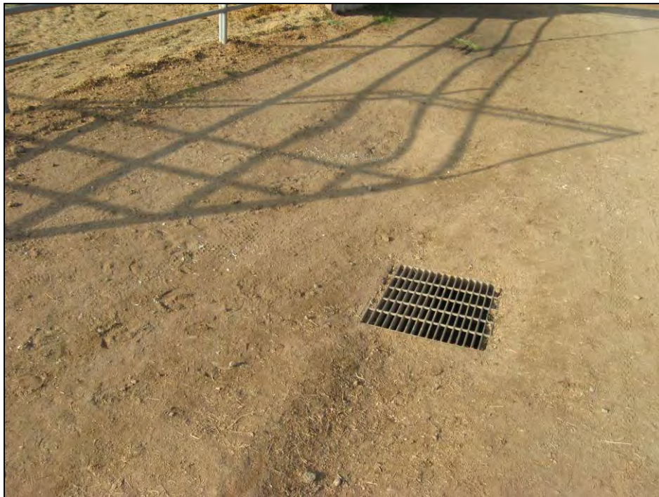
Photograph #10 Two-foot by two-foot storm water inlet on the southeast portion of the Site.
