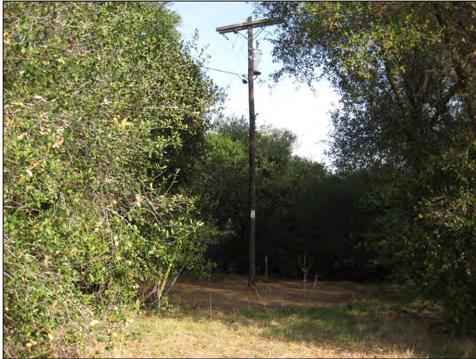
Photograph #17 Pole mounted transformer in the northwestern portion of the Site.
