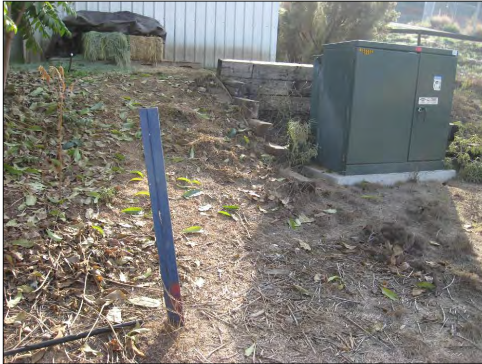
Photograph #11 Pad-mounted electrical transformer and municipal water pipeline marker on the southern portion of the Site.
