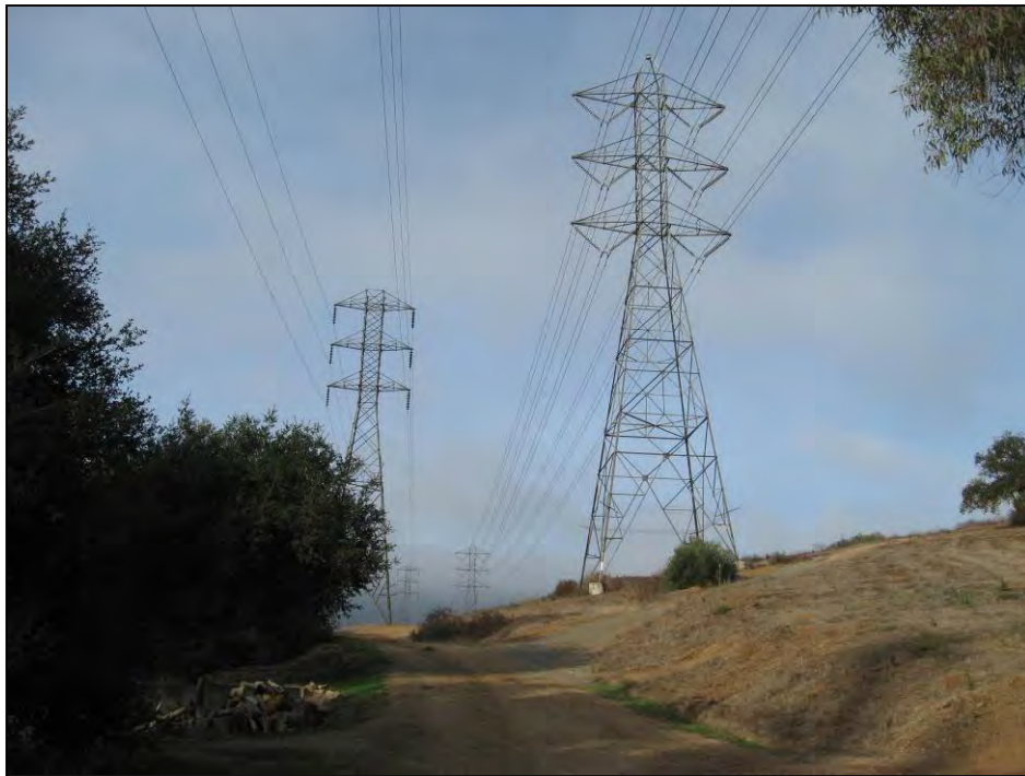
Photograph #16 High tension power lines extending across the south-central portion of the Site.
