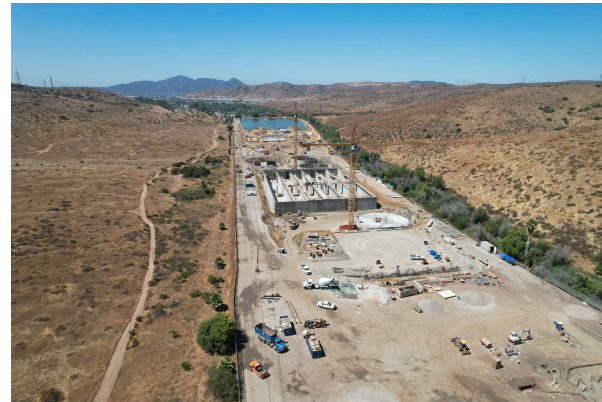
Construction of a water recycling and purification facility near unincorporated El Cajon as part of the East County Advanced Water Purification program
