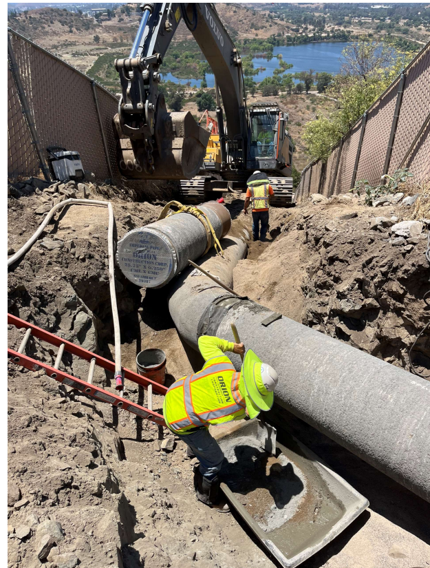
Construction of a water pipeline to Lake Jennings as part of the East County Advanced Water Purification program
